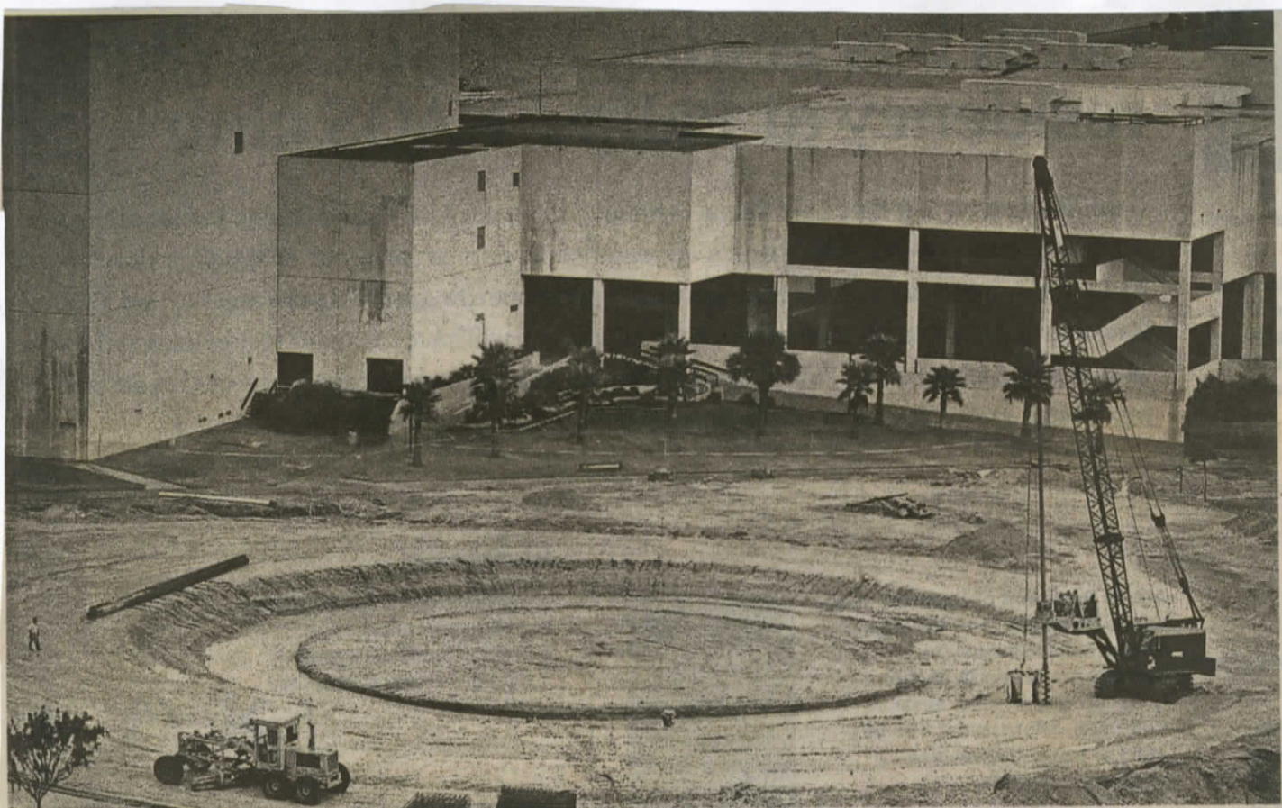
The Watergarden takes shape in front of the Bayfront Plaza Convention Center in Corpus Christi on Aug. 31, 1987.
