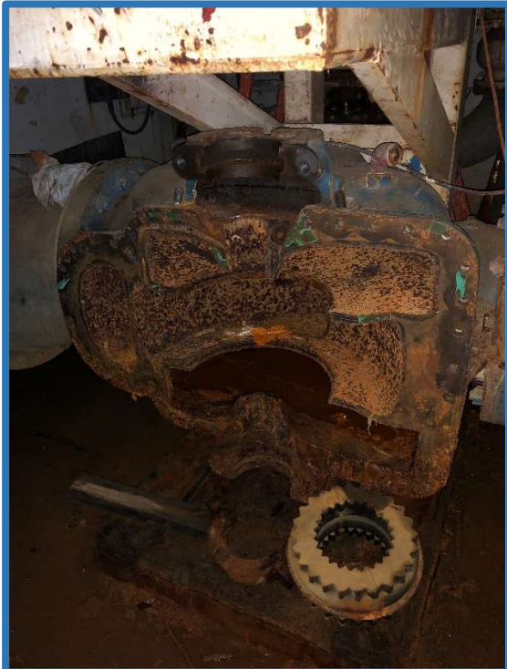
Corroded Main Display Pump
