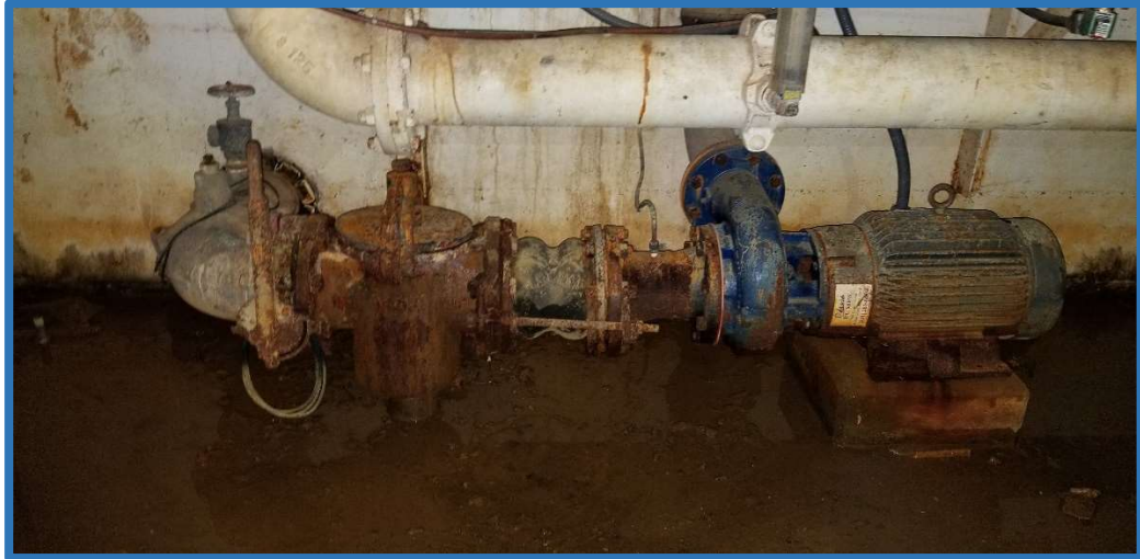
Corroded Sand Filter Pump
