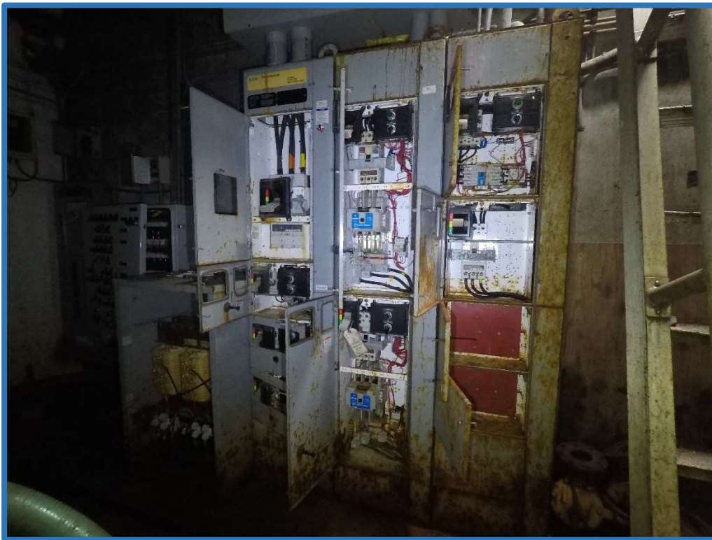
Electrical Control Panel – Corrosion Indicates Water Level
